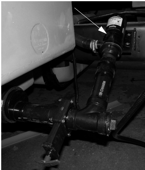
Waste Pump (Located on driver side of coach behind rear wheel) -Typical View
