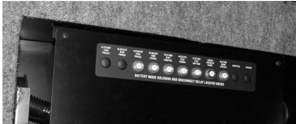
Chassis and House 12V Breakers (Located in passenger side compartment)
