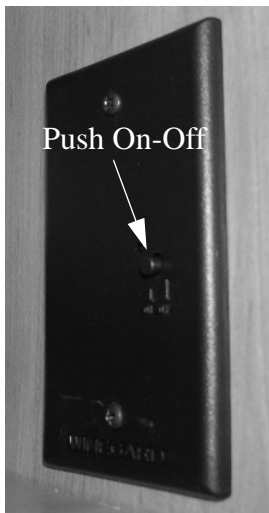
TV Signal Amplifier Power Switch -Typical View
