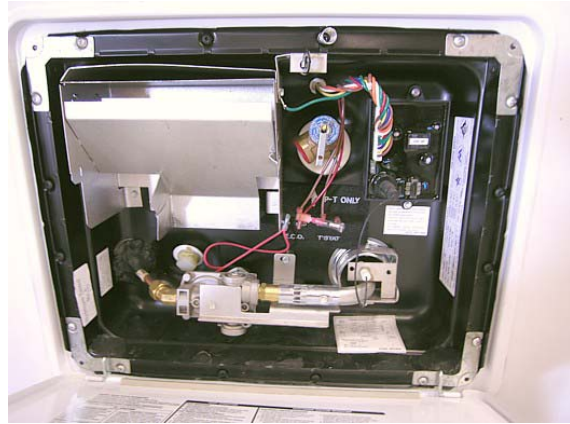
Water Heater Exterior Service Access
