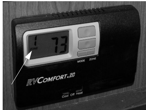
Zone 1 Operation (Living Area/Galley)
