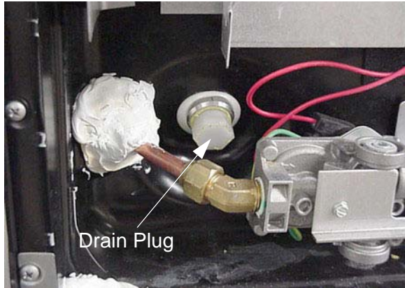
Water Heater Service Access (Located at base of water heater - accessible from outside of coach) -Typical View
