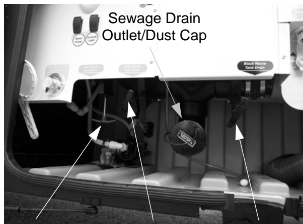
Gray Waste Tank Drain Valve #1 Gray Waste Tank Drain Valve #2 Black Waste Tank Drain Valve
