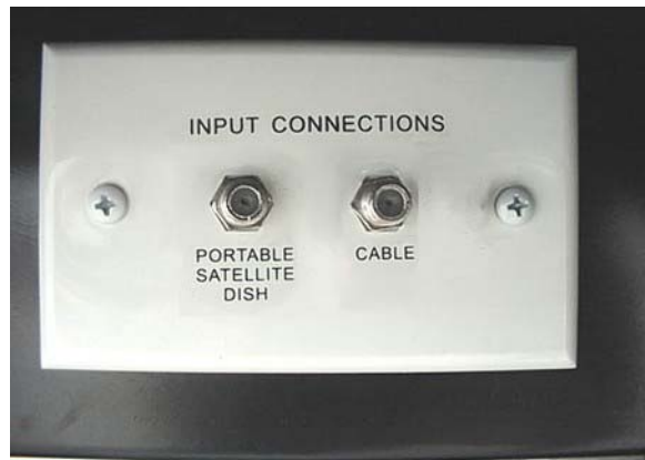
Exterior Connection for Satellite Dish and Cable TV (Located in utility compartment)
