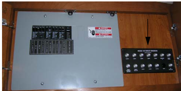
House 12-Volt Circuit Breaker Panel -Typical View
