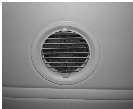
Return Air Vent (Shown with filter installed)
