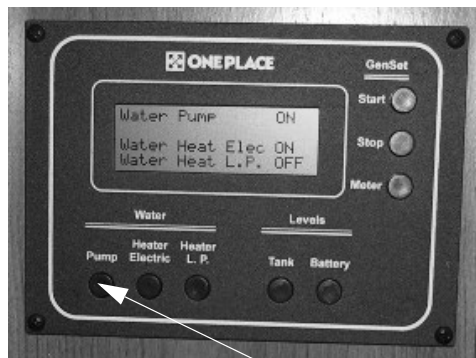
Water Pump Switch
