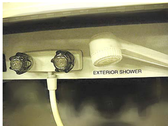
Exterior Shower/Wash Station -Typical View
