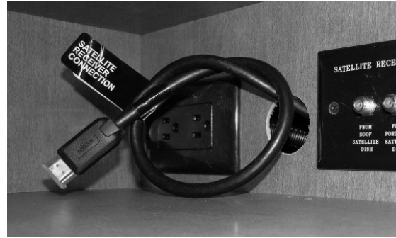
HDMI Cable (Located near entertainment center cabinet) -Typical View
