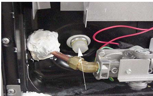
Water Heater Drain Plug (Remove with socket)
