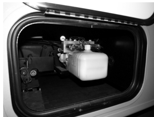
Hydraulic Oil Reservoir (Located in mid-passenger side compartment) -Typical View
