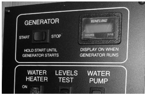
Generator Switch and Hourmeter on monitor panel
