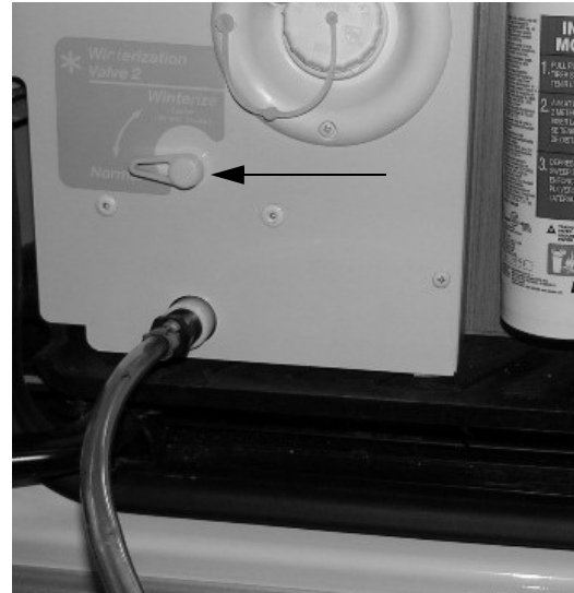
Winterization Valve 2 (Located near sliding entrance door)
