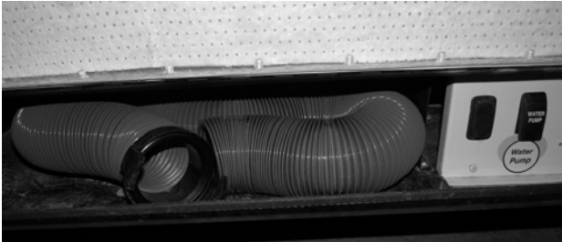
Sewage Drain Hose (Located in water service center)
