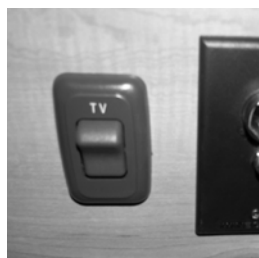
Master 12-Volt Power Switch (Located on underside of cabinet near TV)
