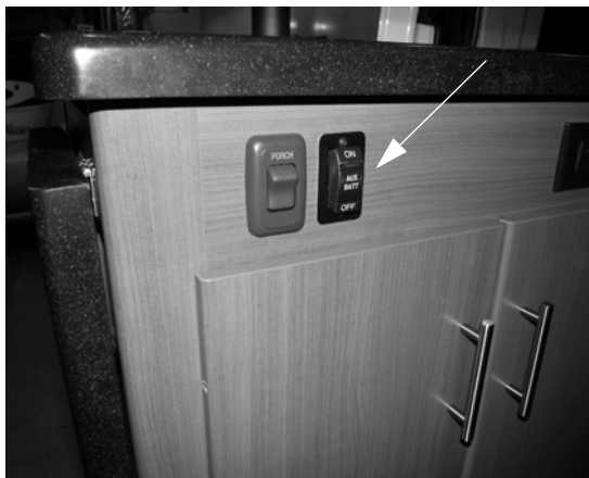
House/Coach Battery Disconnect Switch (Located on front side of galley)
