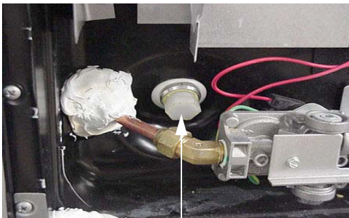
Water Heater Drain Plug (Remove with socket)
