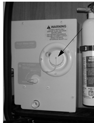
Water Tank Gravity Fill (Located near sliding entrance door) -Typical View
