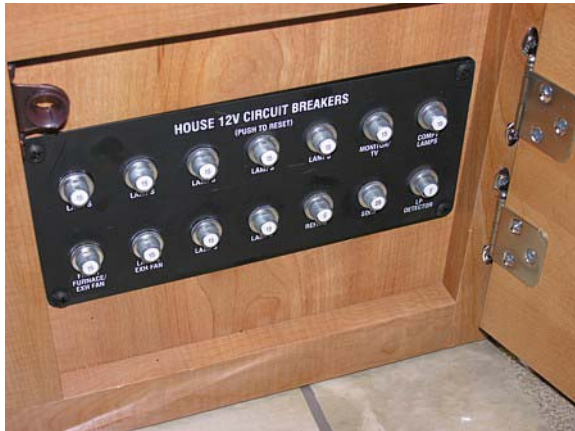
House Circuit Breakers -Typical View
