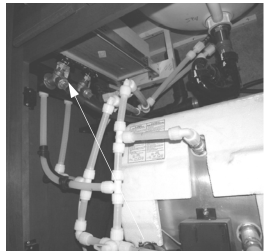
Water Supply Faucets (Located behind water heater - beneath bedroom lavatory cabinet)
