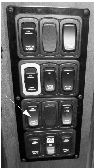
Compartment Lights Switch (Located near entrance door) -Typical View
