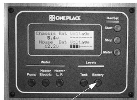
Battery Levels Switch
