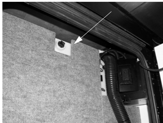
Gravity Fill Port (Located in first passenger side compartment)
