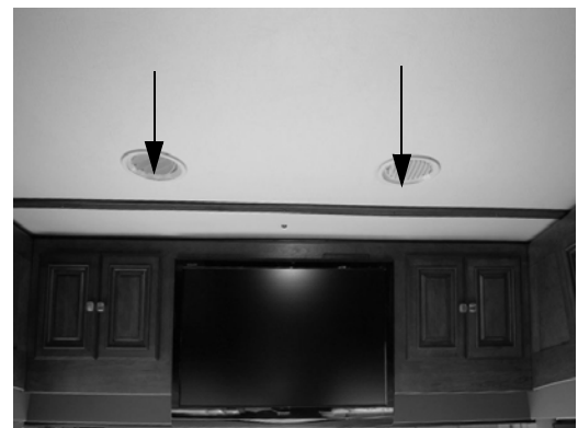
Supply/Return Air Vents (Located throughout the ceiling of the coach) -Typical View
