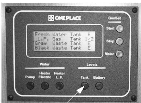
Tank Levels Switch
