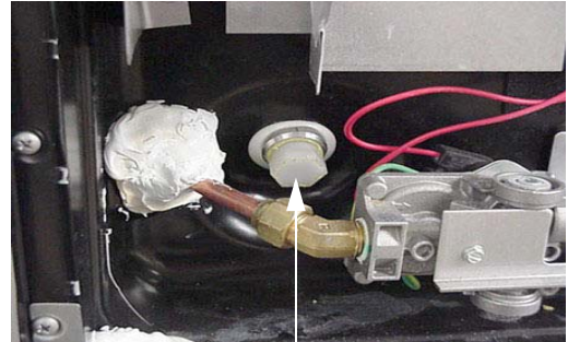
Water Heater Drain Plug (Remove with socket)
