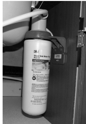
Cold Water Filter Assembly (Located below galley sink)
