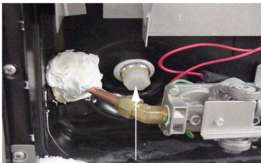
Water Heater Drain Plug (Remove with socket)
