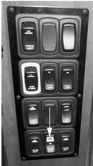
Entry Step Switch (Located near the entrance door) -Typical View
