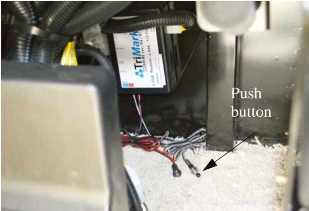
Keyless Entry Control Box (Located below driver side dash) -Typical View
