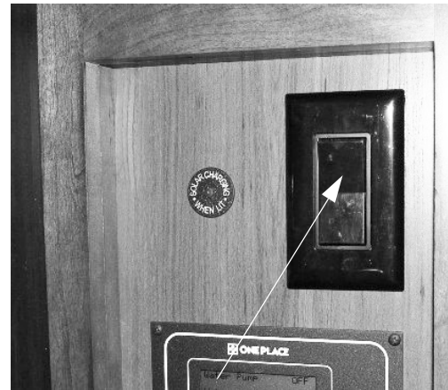
Diesel Engine Heater Switch (Located near monitor panel) -Typical View
