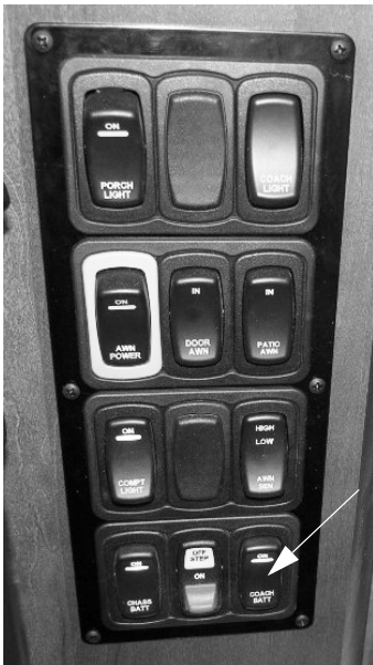
House/Coach Battery Disconnect Switch (Located near entrance door) -Typical View
