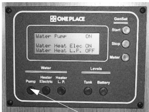
Water Pump Switch
