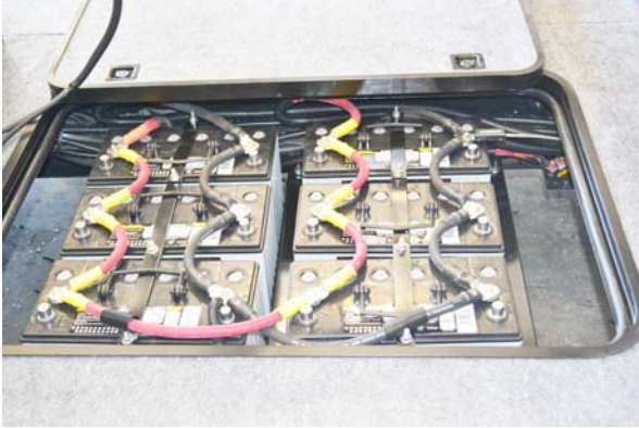
House/Coach Batteries (Shown with access cover removed) -Typical View
