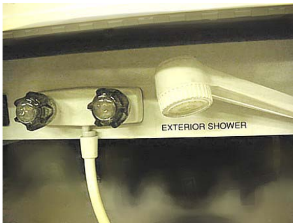
Exterior Shower/Wash Station -Typical View
