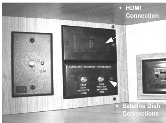
Interior Satellite Dish and HDMI Connections (Located near entertainment center cabinet) -Typical installation shown
