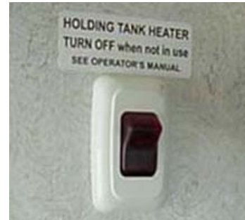
Holding Tank Heater Switch -Typical installation shown
