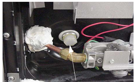
Water Heater Drain Plug (Remove with socket)
