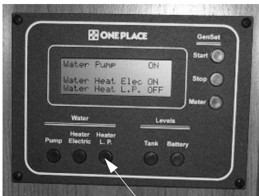
Propane Gas Water Heater Switch (Located on OnePlace® monitor panel)
