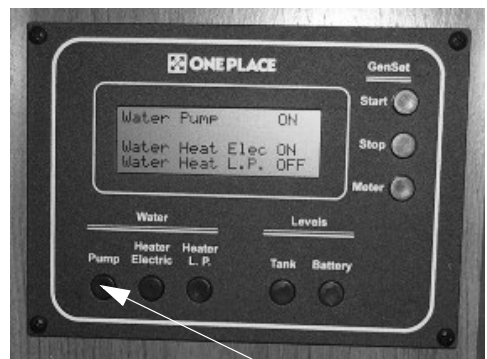
Water Pump Switch
