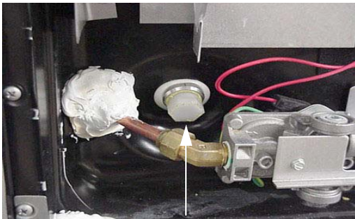
Water Heater Drain Plug (Remove with socket)
