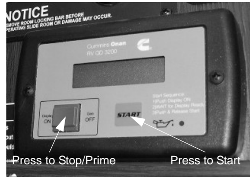
Diesel Generator Start/Stop Buttons (Located near monitor panel) -Typical View
