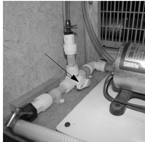
Winterization Valve -Typical View
