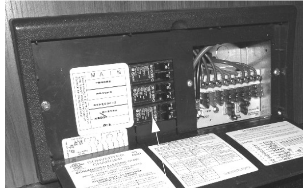
120-Volt Circuit Breakers -Typical View
