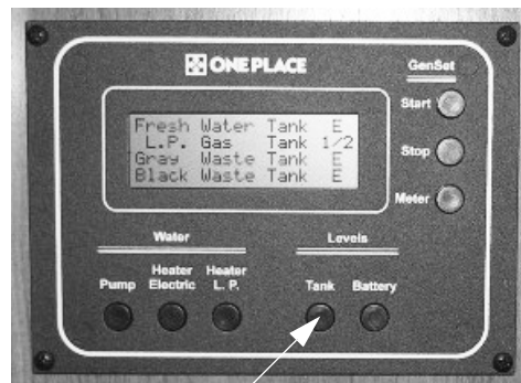
Tank Levels Switch
