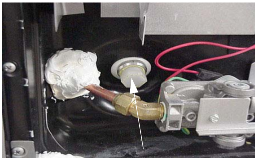
Water Heater Drain Plug (Remove with socket)
