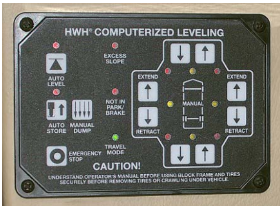
Leveling System Control Panel (Located near entrance door)
