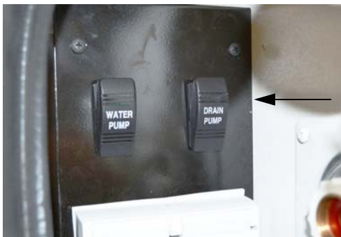
Waste Pump Switch (Located in water service center)
