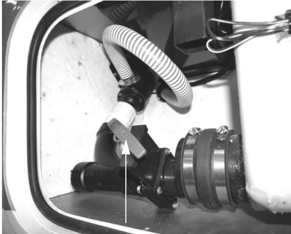
Gray Waste Tank Drain Valve (Located in driver side compartment behind rear wheel)
