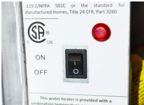
Water Heater (Tankless) Power Switch
