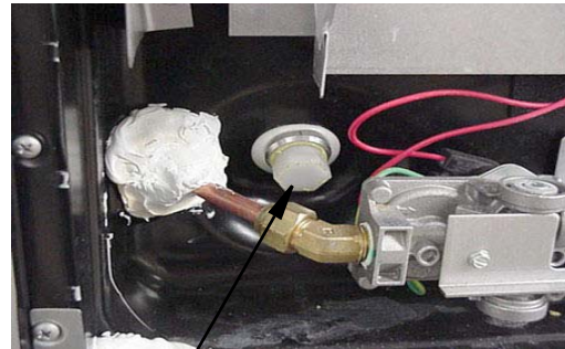
Water Heater Drain Plug (Remove with socket)
