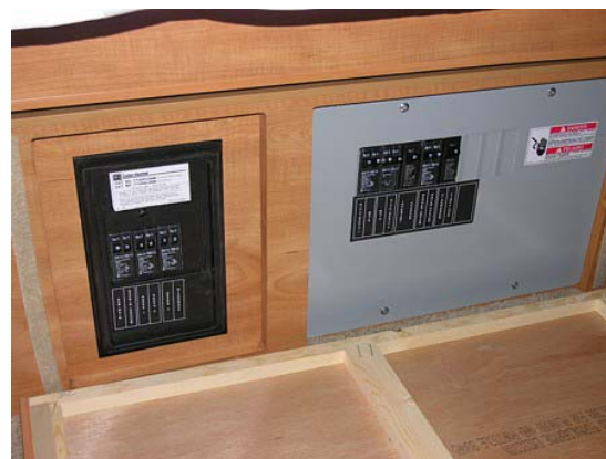
House Circuit Breakers -Typical Installation
