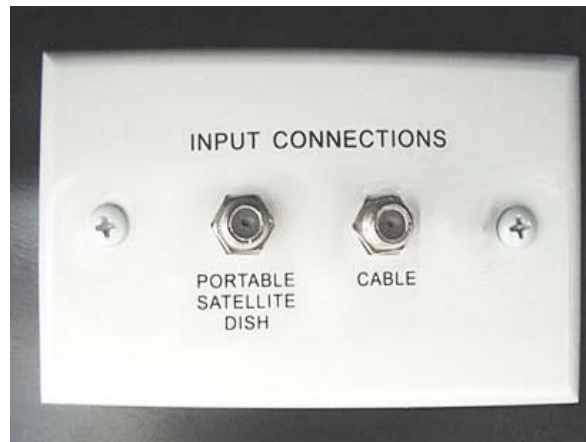
Exterior Connection for Satellite Dish and Cable TV (Located in the shoreline compartment)
