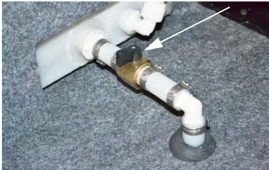
Water Tank Drain Valve (Located in the third passenger side compartment) -Typical View
