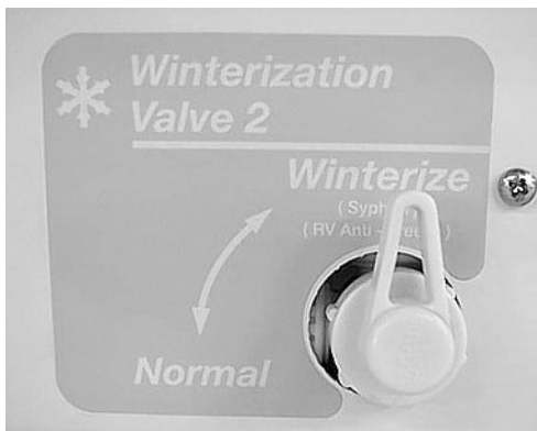
Winterization Valve 2 (Located near water pump - second compartment on driver side of coach)
