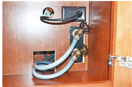
Water Supply Faucets (Located inside cabinet above washer) -Typical View
