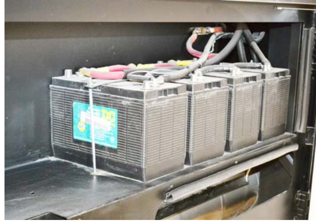
House/Coach Batteries (Located in the rear passenger side compartment.)
