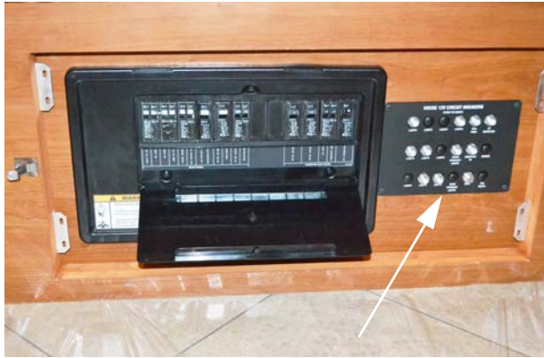
House Circuit Breakers -Typical View
