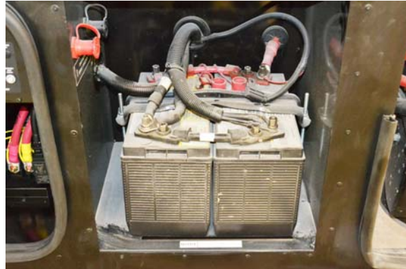
Chassis Batteries (Located in a rear driver side compartment) -Typical View
