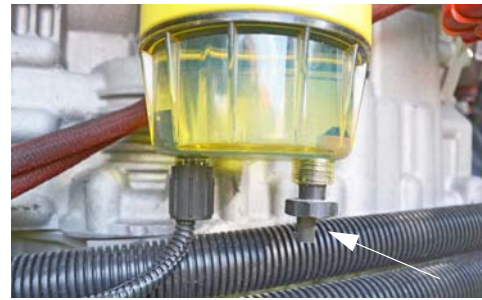
Fuel/Water Separator Drain Valve (Located on bottom end of separator) -Typical View
