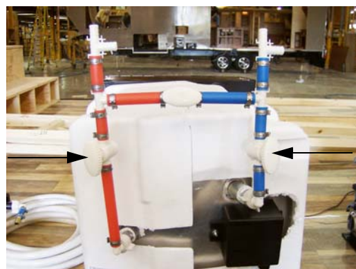
Water Heater Bypass Valves
