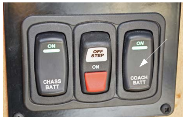
House/Coach Battery Disconnect Switch (Located near entrance door) -Typical View
