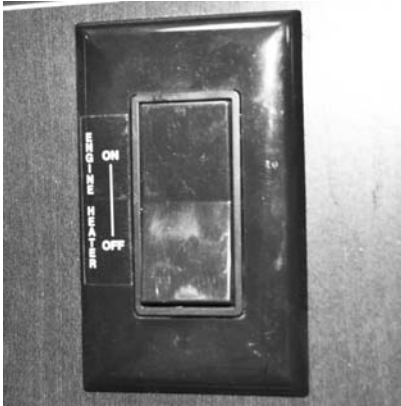
Diesel Engine Heater Switch (Located near monitor panel) -Typical View
