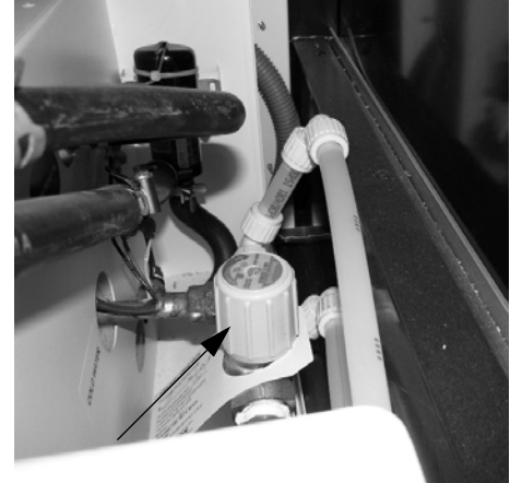
Hydronic Heating System Tempering Valve (Located on back side of the Aqua-Hot unit)
