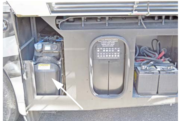
Diesel Exhaust Fluid Fill Tank (Located in driver side compartment behind the rear wheel) -Typical View
