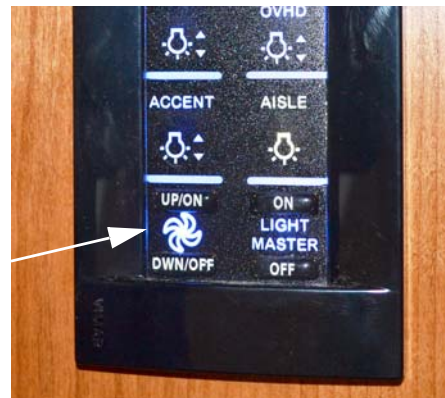
Power Roof Ventilator Switch
