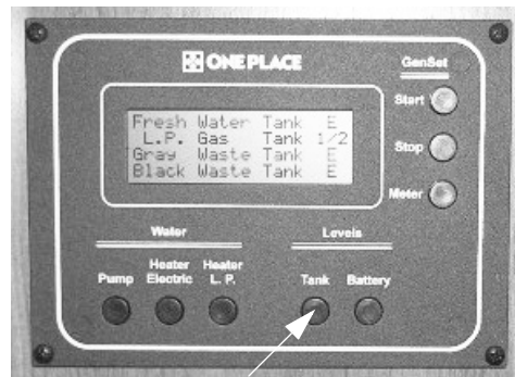
Tank Levels Switch
