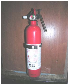
Fire Extinguisher (Typical installation - your coach may vary according to model and floorplan)
