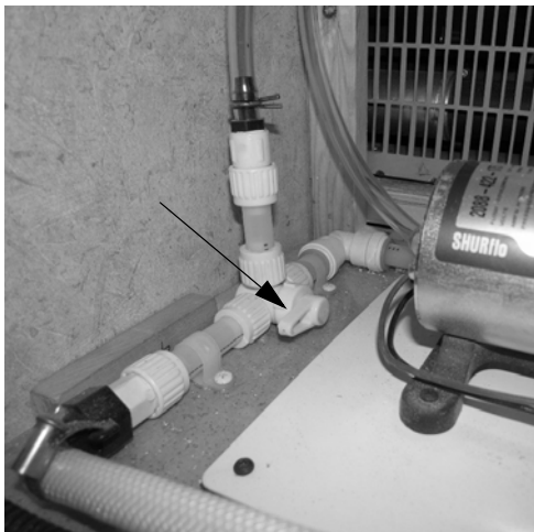
Winterization Valve -Typical View
