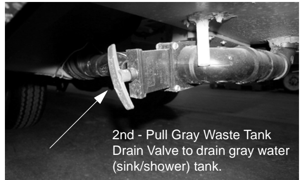
Gray Waste Tank Drain Valve (Located underneath driver side rear compartment) -Typical View
