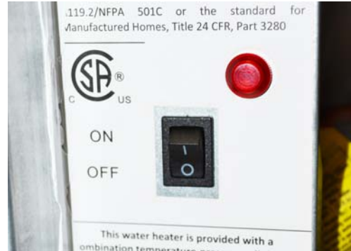
Water Heater (Tankless) Power Switch
