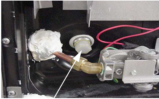
Water Heater Drain Plug (Remove with socket)
