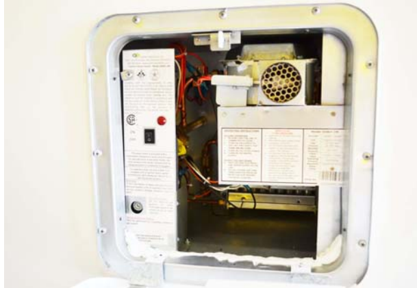
Water Heater Exterior Service Access -Typical View
