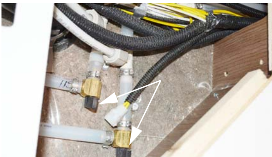
Waterline Drain Valve
