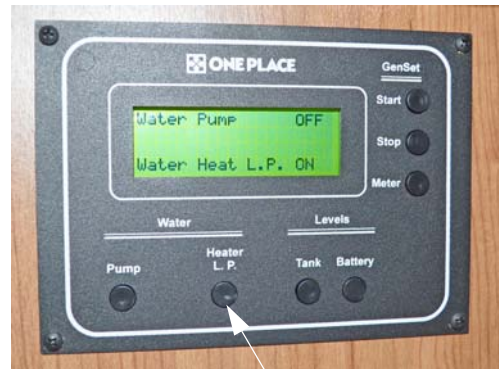
LP Gas Water Heater Switch
