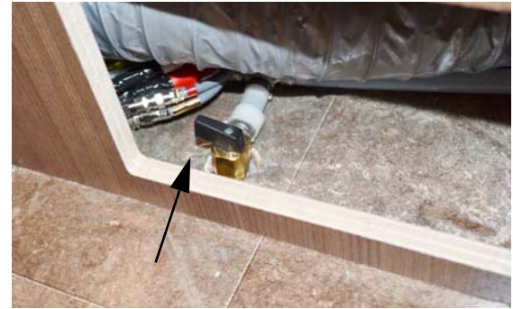
Water Tank Drain Valve
