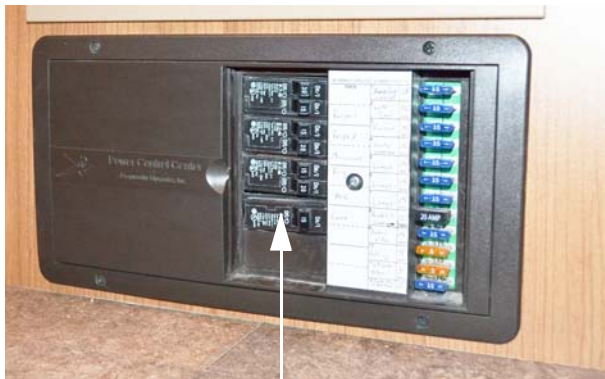
120-Volt Circuit Breakers -Typical View
