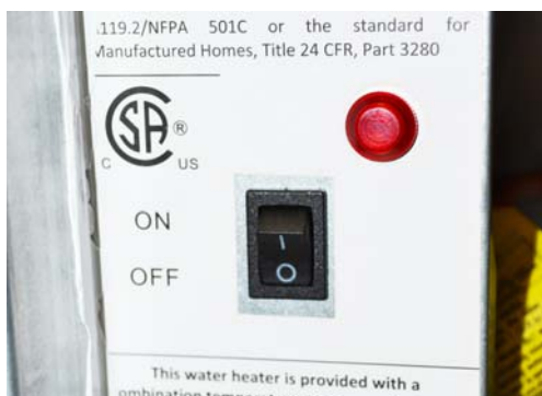
Water Heater (Tankless) Power Switch
