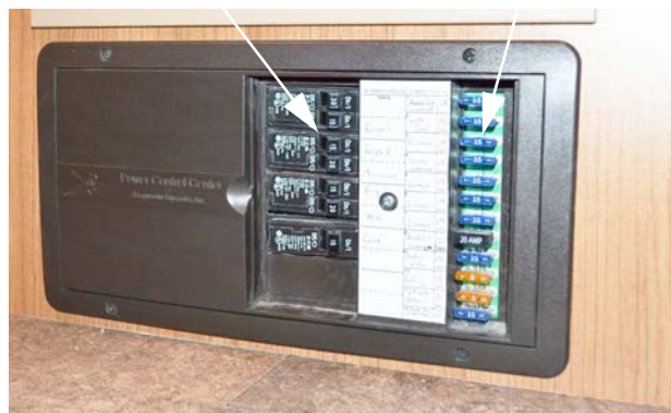
Power Center (Converter) -Typical View
