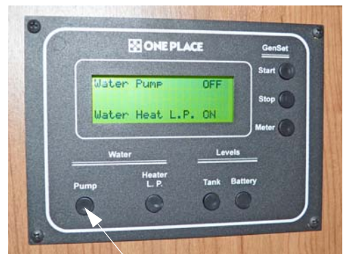
Water Pump Switch
