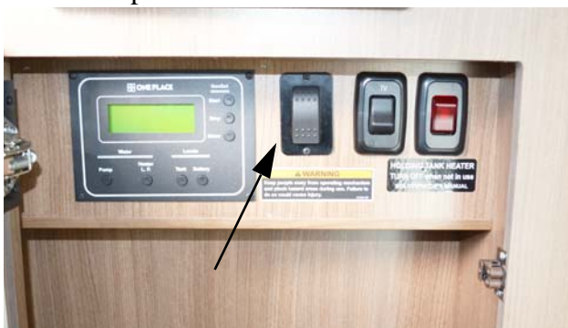
Loft Bed Switch (Located inside cabinet near the entrance door)
