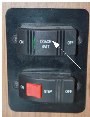
House/Coach Battery Disconnect Switch (Located near entrance door or end of galley, depending on model) -Typical View
