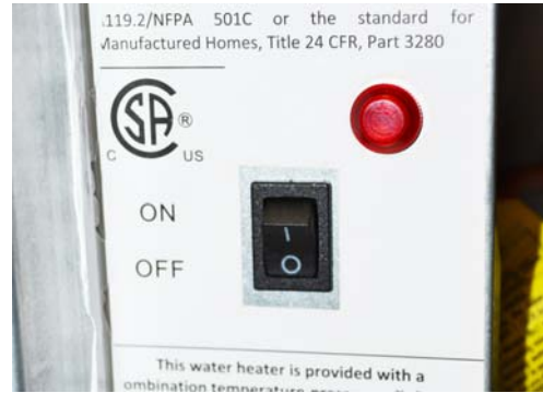
Water Heater (Tankless) Power Switch
