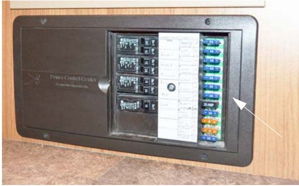
House 12-Volt Fuses (Located on right-hand side of Power Converter) -Typical View
