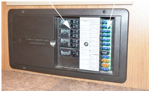
Power Center (Converter) -Typical View
