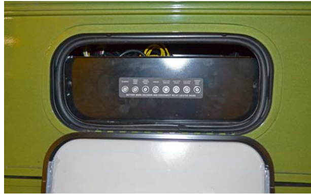
Automotive Chassis and House 12-Volt Circuit Breakers (Located inside a driver side compartment) -Typical View
