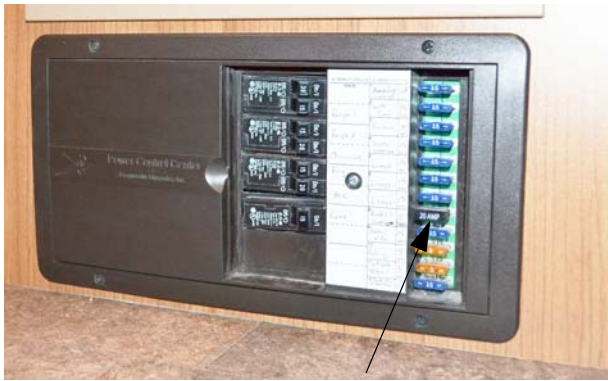
House 12-Volt Fuses (Located on Power Converter) -Typical View
