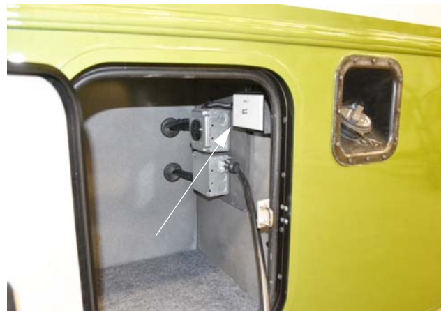
Cable TV Connection (Located in an exterior driver side compartment) -Typical installation shown
