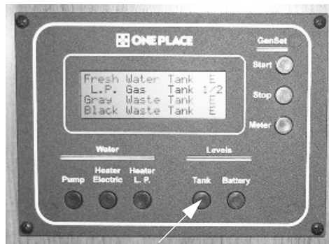
Tank Levels Switch
