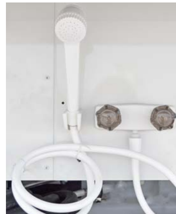
Exterior Shower/Wash Station -Typical View
