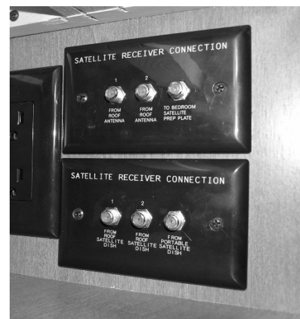
Interior Satellite Dish Connections (Located in the entertainment center cabinet) -Typical View
