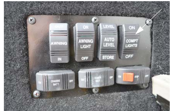
Compartment Lights Switch (Located near entrance door) -Typical View
