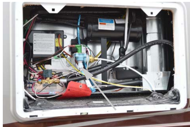
Ice Maker Water Supply Connection (Located in refrigerator service access compartment on outside of coach) -Typical View
