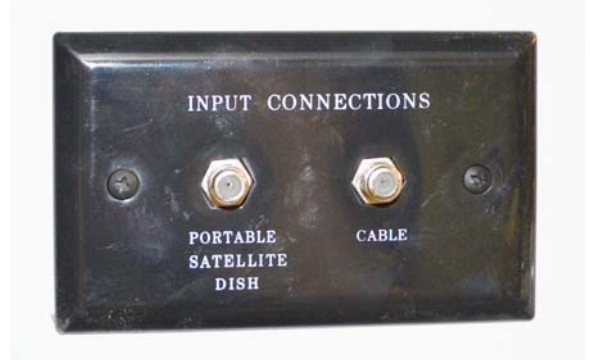
Exterior Connection for Satellite Dish and Cable TV (Located in utility compartment) -Typical View
