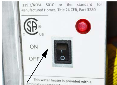
Water Heater Power Switch (Push up to turn ON)
