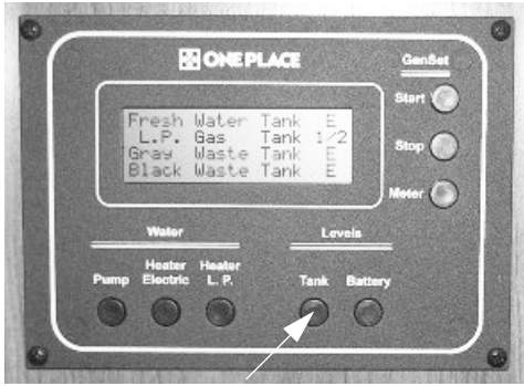
Tank Levels Switch
