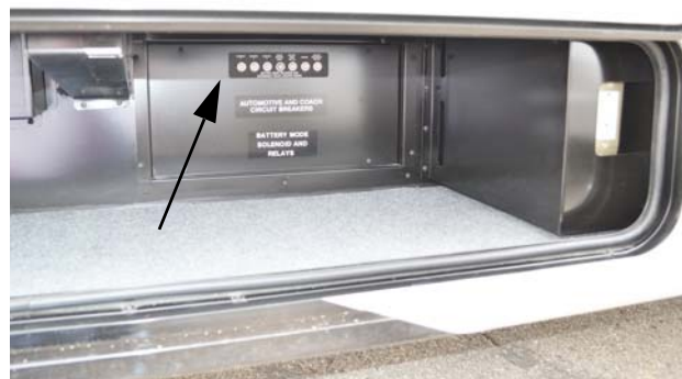
Automotive Chassis and House 12-Volt Circuit Breakers (Located inside passenger compartment) -Typical View
