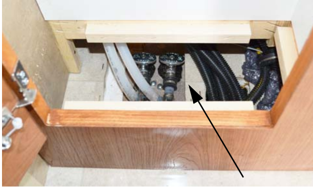
Waterline Drain Valves -Typical installation shown
