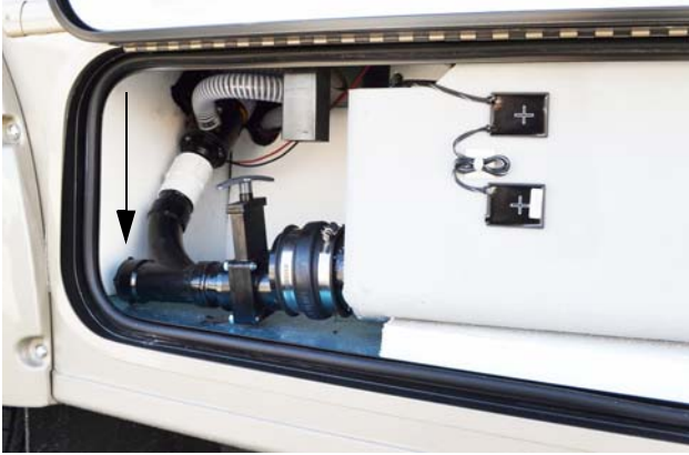
Waste Pump Drain (Located in driver side compartment behind rear wheel)
