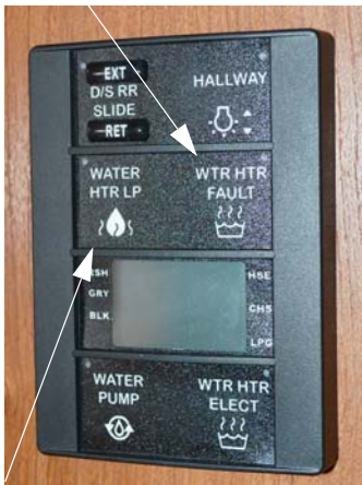
Propane Gas Water Heater Switch (Located on Systems Monitor Panel) -Typical View
