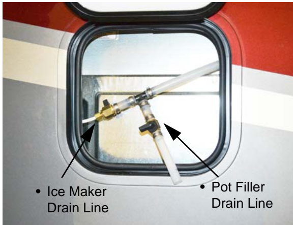
Pot Filler and Ice Maker Drain Line (Located in exterior Residential Refrigerator service compartment)
