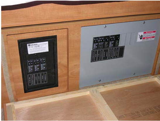
House Circuit Breakers -Typical Installation
