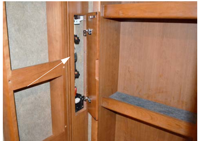
Water Supply Faucets (Located inside wardrobe behind access door)
