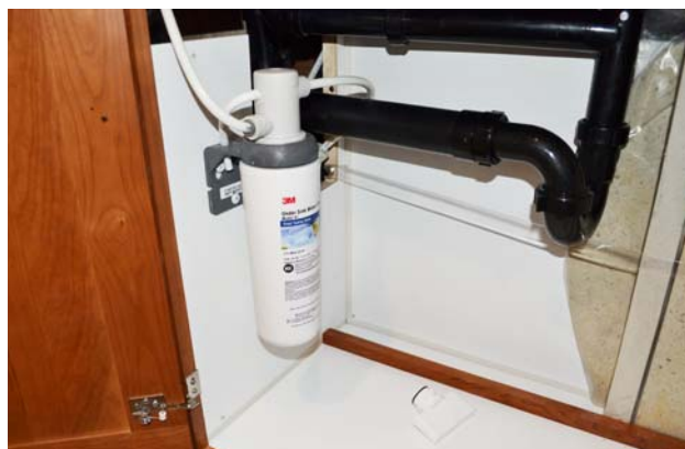
Galley Filtered Cold Water Faucet/ Ice Maker Filter Assembly (Located below galley sink) -Typical View
