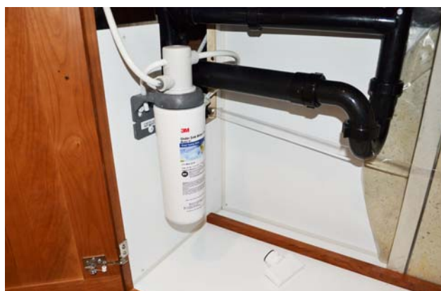
Galley Filtered Cold Water Faucet/ Ice Maker Filter Assembly (Located below galley sink) -Typical View
