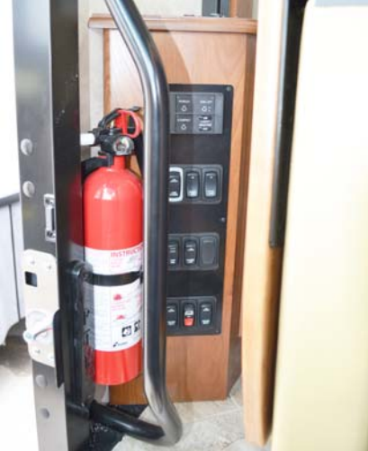
Fire Extinguisher (Located near entrance door) -Typical installation shown
