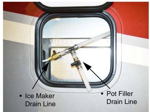
Pot Filler and Ice Maker Drain Line (Located in exterior Residential Refrigerator service compartment)
