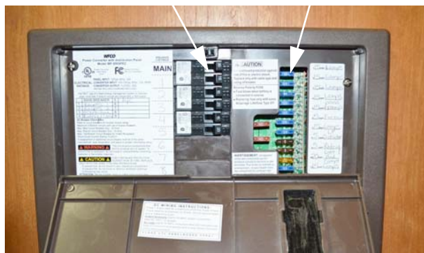
Power Center (Converter) -Typical View
