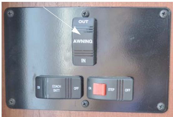
Power Awning Switch (Located near entrance door) -Typical View
