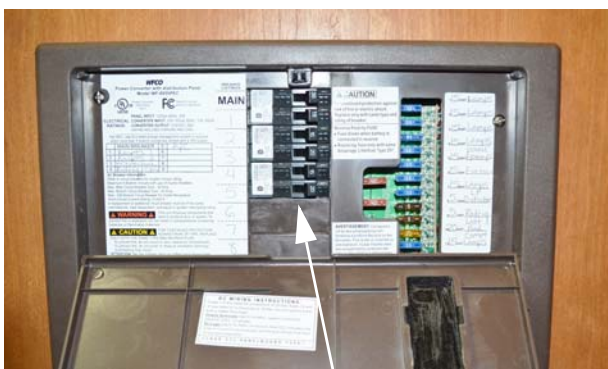
120-Volt House Circuit Breakers -Typical View
