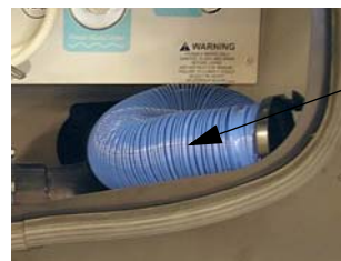
Sewage Drain Hose -Typical View
