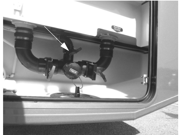
Black Waste Tank Drain Valve #2 (Front) (Located in water service center) -Typical View
