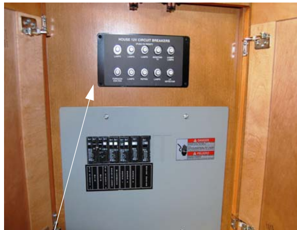
House 12-Volt Circuit Breakers (Models 35B, 35F, and 36Y) -Typical View
