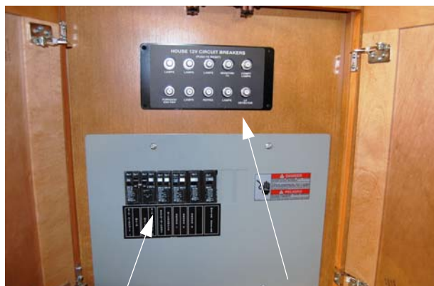
120-Volt House Circuit Breakers
