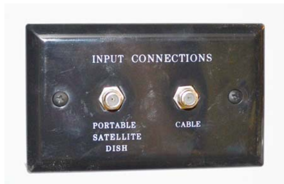
Satellite Dish and Cable TV Connections (Located in utility compartment or water service center) -Typical View
