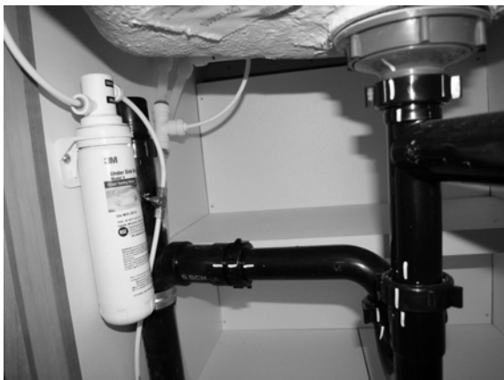
Ice Maker Water Filter Assembly (Located below galley sink)
