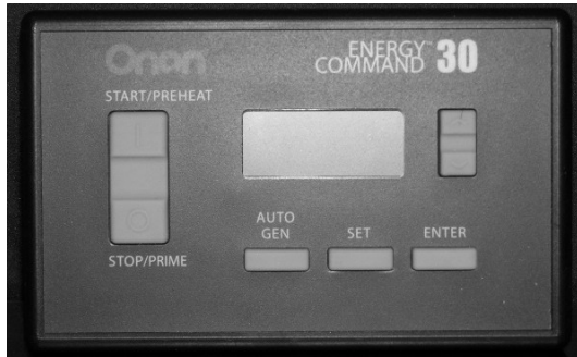
AGS Control Pad (Located near monitor panel)
