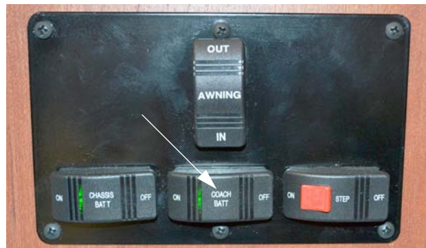
House/Coach Battery Disconnect Switch (Located near entrance door) -Typical View
