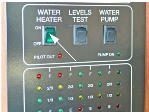
Gas Water Heater Switch (Located on Systems Monitor Panel)
