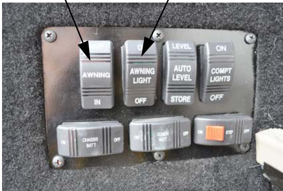
Awning Control Switch and Awning Light Switch (Located near entrance door) -Typical View
