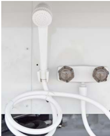
Exterior Shower/Wash Station -Typical View
