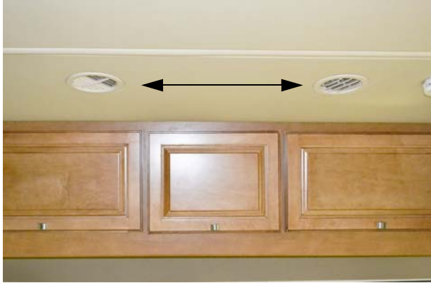
Supply/Return Air Vents (Located throughout the ceiling of the coach) -Typical View
