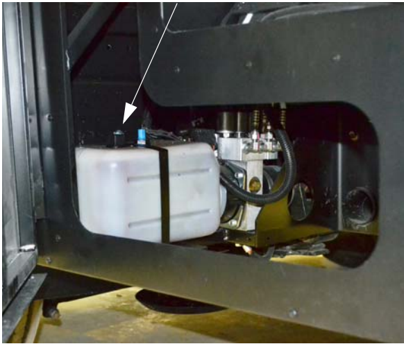
Hydraulic Oil Reservoir (Located behind driver side front tire) -Typical View
