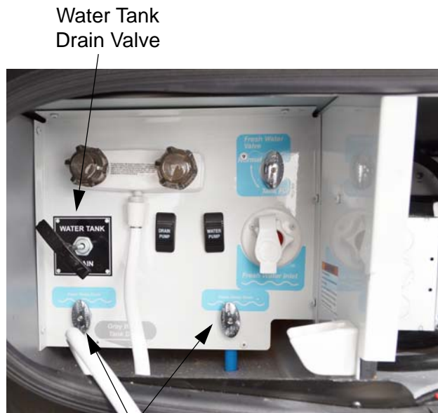
Water Tank Drain Valve Waterline Drain Valves -Typical View
