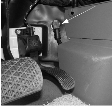
Chassis Battery Connector (Located to the right of the accelerator pedal)
