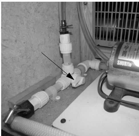
Winterization Valve -Typical View
