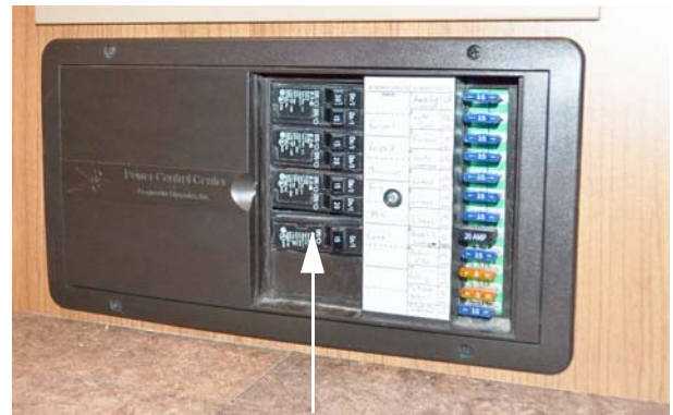
120-Volt Circuit Breakers -Typical View
