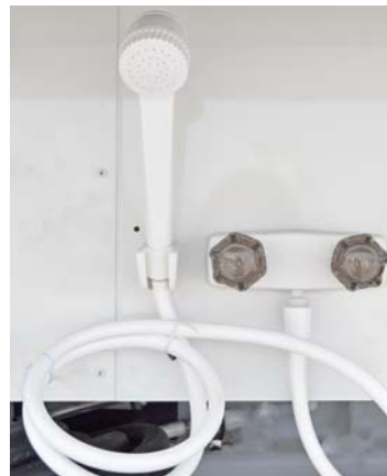
Exterior Shower/Wash Station -Typical View
