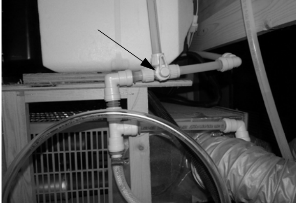
Water Heater Bypass Valve
