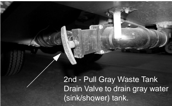
Gray Waste Tank Drain Valve (Located underneath driver side rear compartment) -Typical View
