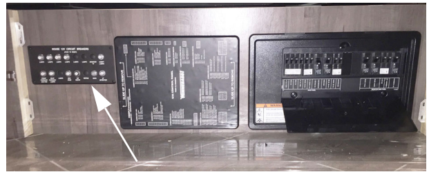
House Circuit Breakers -Typical View
