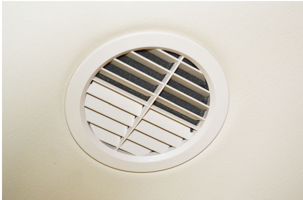
Return Air Vent (Shown with filter installed) -Typical View
