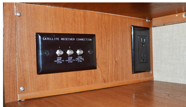
Interior Satellite Dish Connections (Located in the entertainment center cabinet) -Typical View
