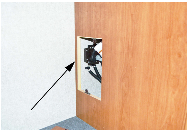
Water Supply Faucets (Located behind access panel inside wardrobe) *Model 38F
