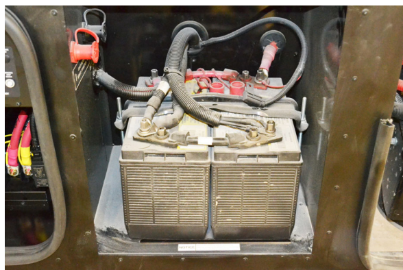
Chassis Batteries -Typical View
