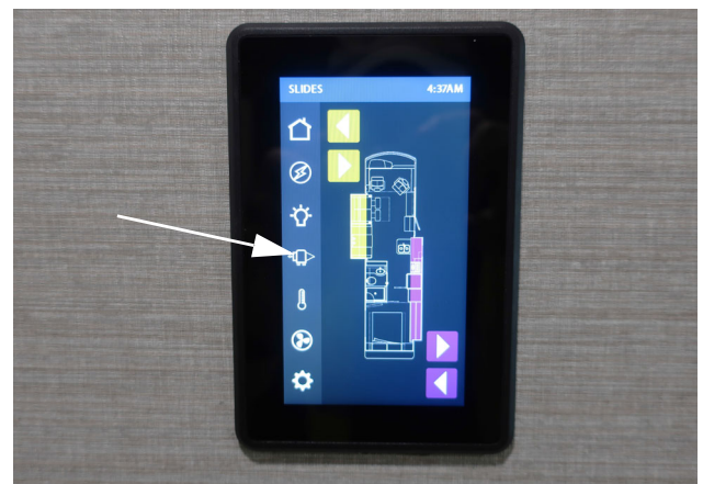
Slideout Switch (Located on Multiplex Monitor Panel) -Typical View
