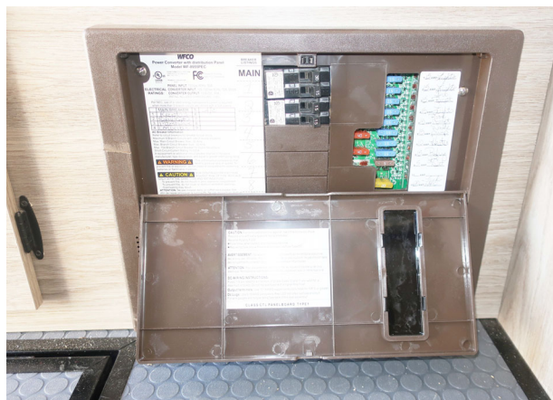
120-Volt Circuit Breakers -Typical View
