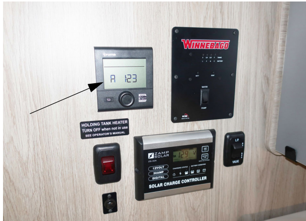
Water heater controls on Systems Monitor Panel -Typical View
