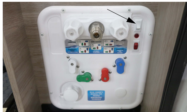
Pump switch -Typical View
