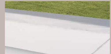
One-year-old Winnebago Industries fiberglass roof
