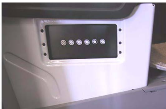
Chassis and House 12V Breakers on side of passenger seat base toward door (shown w/cover off)
