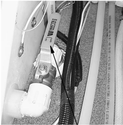
Water Tank Drain Valve (Typical)
