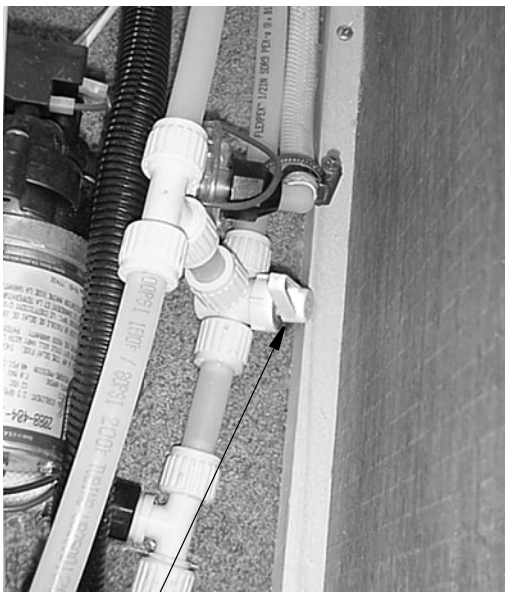
Water Heater Bypass Valve (Typical)
