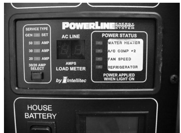
EMS Display on Monitor Panel
