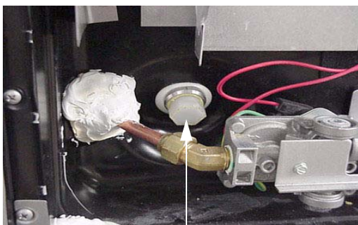
Water Heater Drain Plug (Remove with socket)
