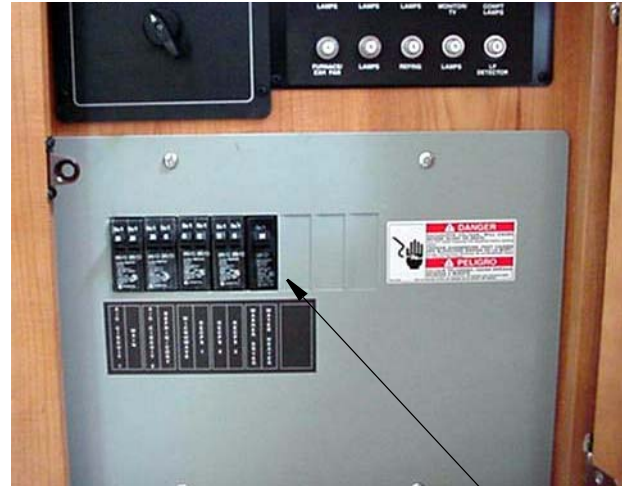
120-Volt House Circuit Breakers
