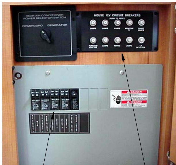
120-Volt House Circuit Breakers
