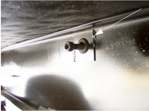
Manual Override, Requires a 3/4 inch wrench
