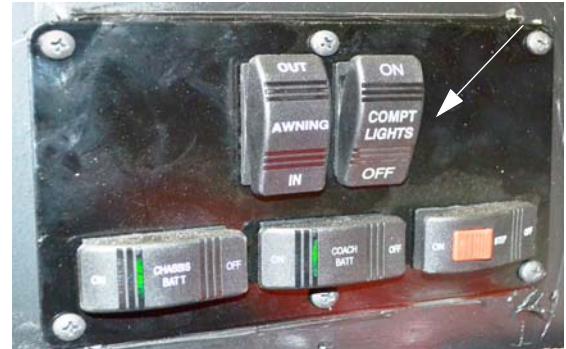
Compartment Lights Switch (Located near entrance door) -Typical View
