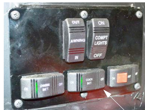
House/Coach Battery Disconnect Switch (Located near entrance door) -Typical View
